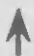
A nearly completed roof, seen from within Tank 910. Sunshine penetrates from some sections of the roof that are still not covered.
